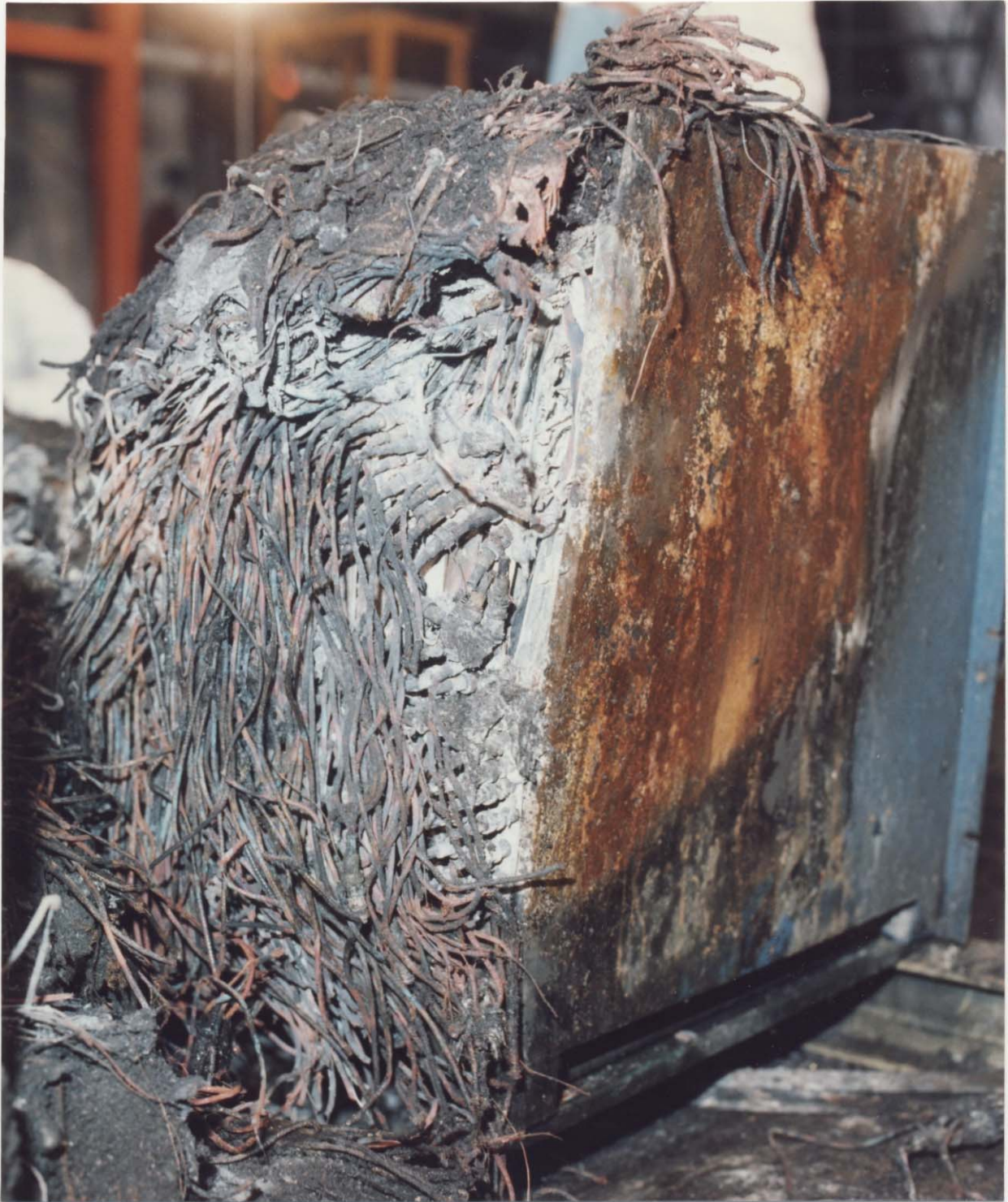
Figure 23. Extensive fire damage to rear of MF7. The top has been mechanically damaged from weight of fallen cables.
