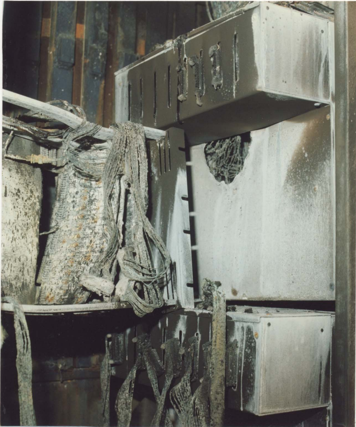
Figure 27. Interior of upstream side of dynode sum box. Connectors handled immediately prior to fire are on lower chassis box. Suspect connector is third from outside.
