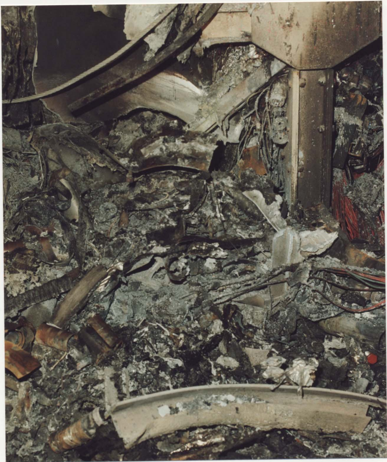
Figure 19. Rubble pile below the IEC containing damaged PMT parts, aluminum frame pieces, and burnt cables.
