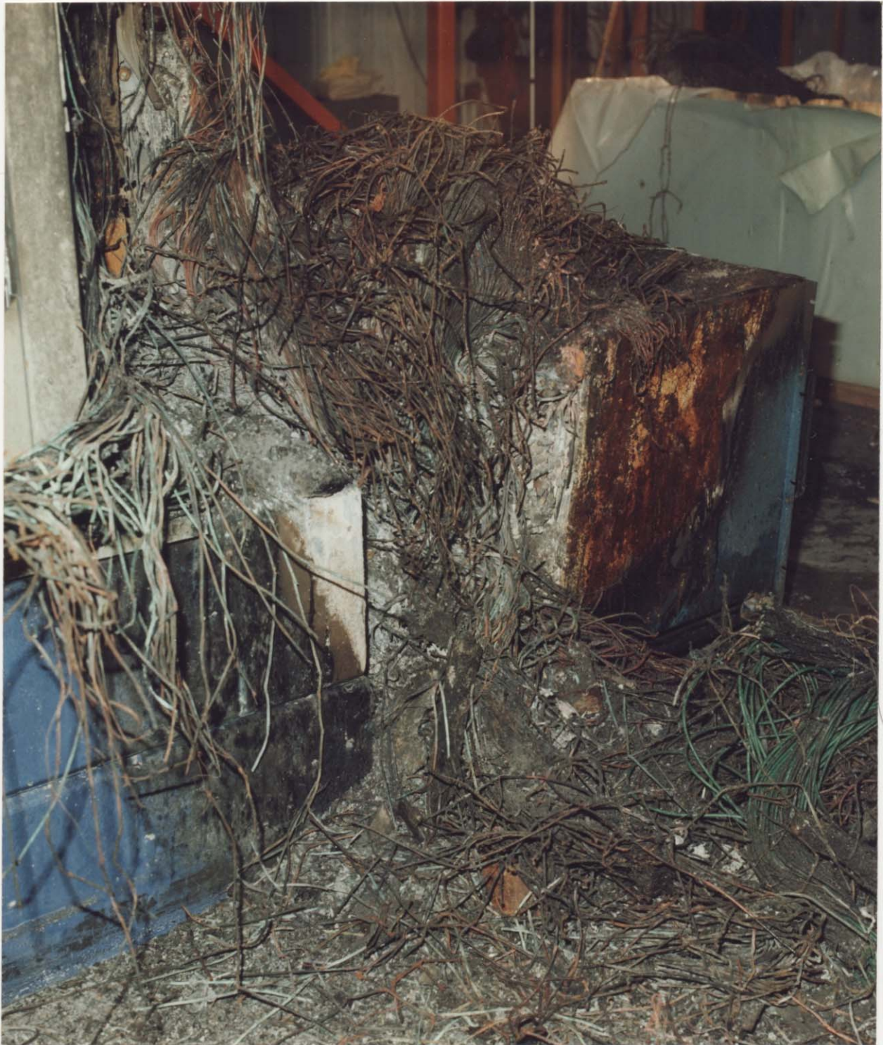
Figure 20. "V" pattern on southwest HC shielding block support and MF7 caused by burning cables.
