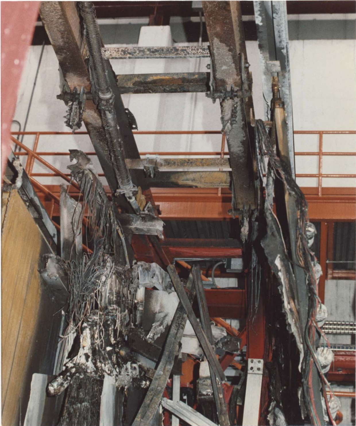
Figure 11. Damage to upper portion of IEC aluminum framework and support structure. Note remnants of HxV.
