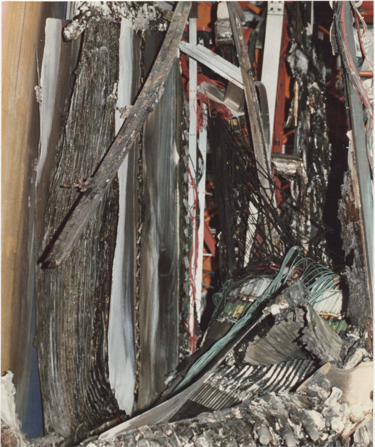
Figure 17. View of damage to IEC looking east prior to removal of HxV and P4. IEC third module is still hanging from aluminum framework and second module is in foreground.
