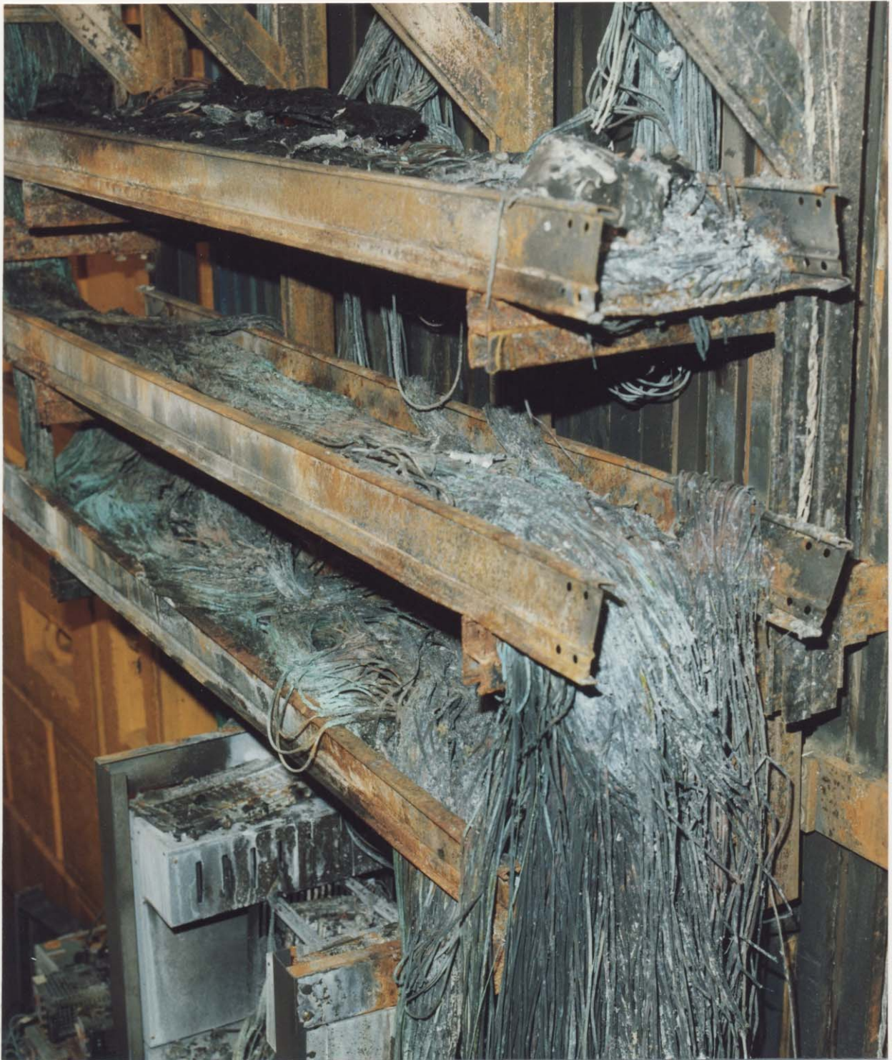
Figure 22. Fire damage to cables in trays on west side of HC.
