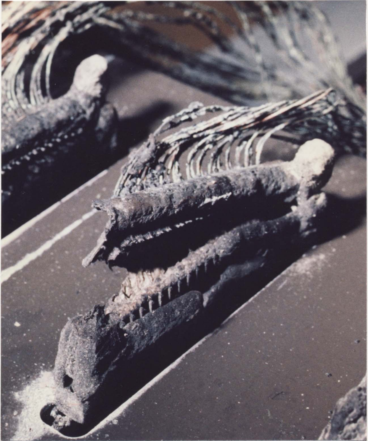
Figure 28. Closeup of suspect connector on lower upstream chassis box. Note lack of plastic on right side of pins.
