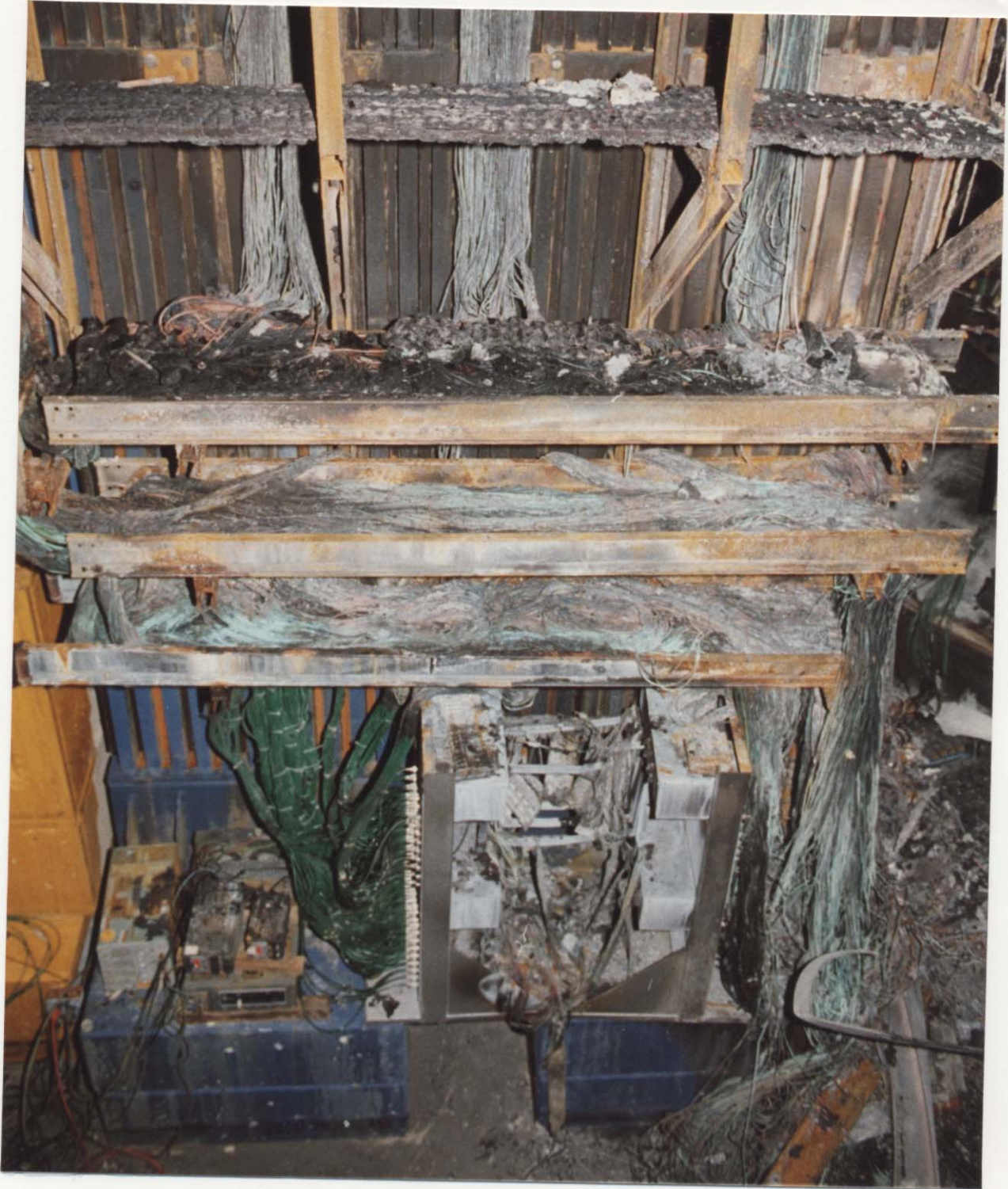
Figure 21. Fire damage to west side of HC.
