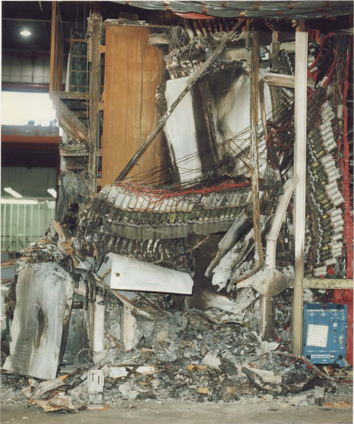
Figure 16. Upstream view of IEC with HxV removed. MF6 is clearly visible on lower right while MF7 is buried under rubble at lower left. Note undamaged cables along east side.
