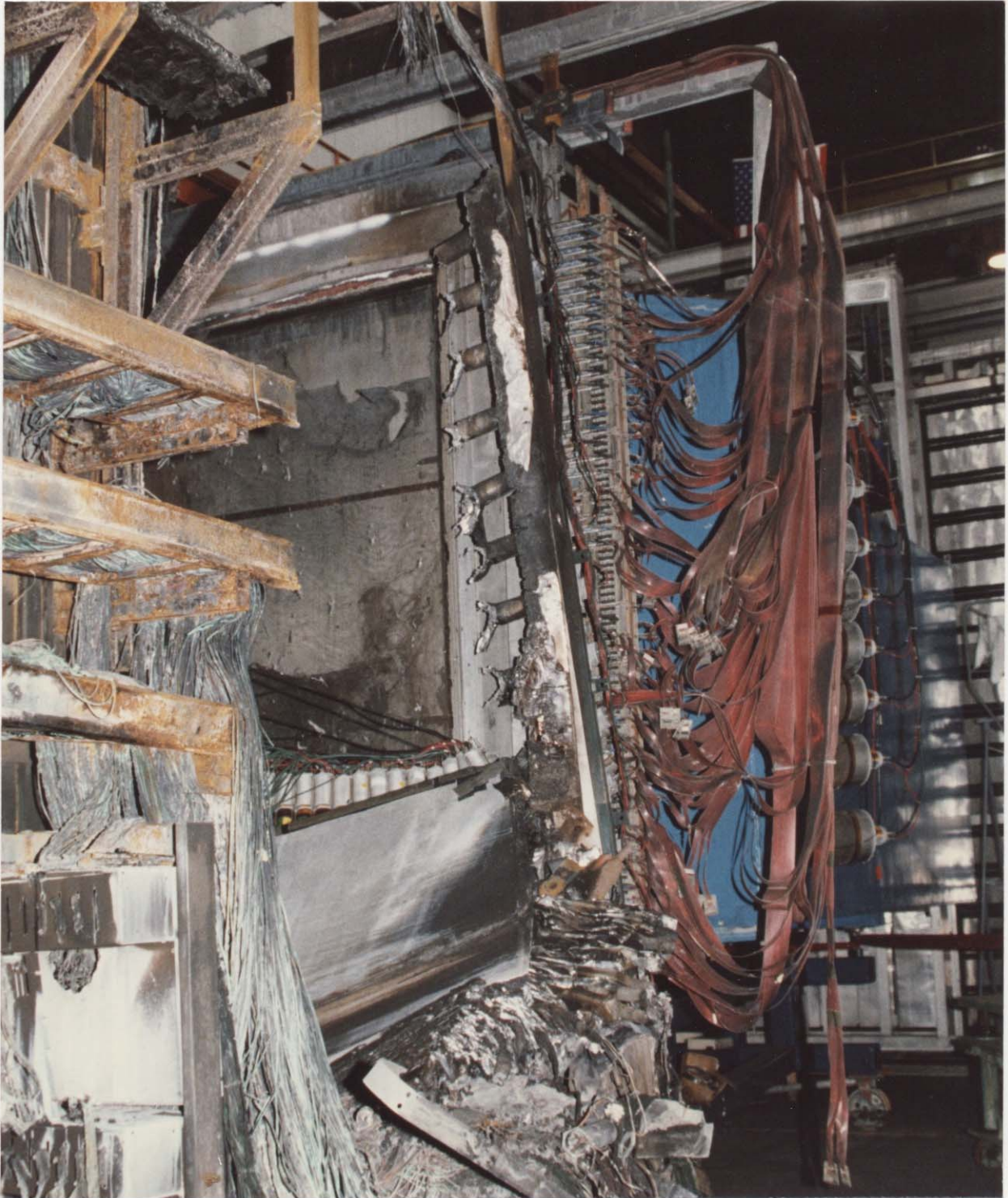
Figure 12. Damage to dynode sum box (with hole burnt through south panel) and IEC second module, remnants of west side of HxV, and damage to P4. Note minor damage to P4 ribbon cables.
