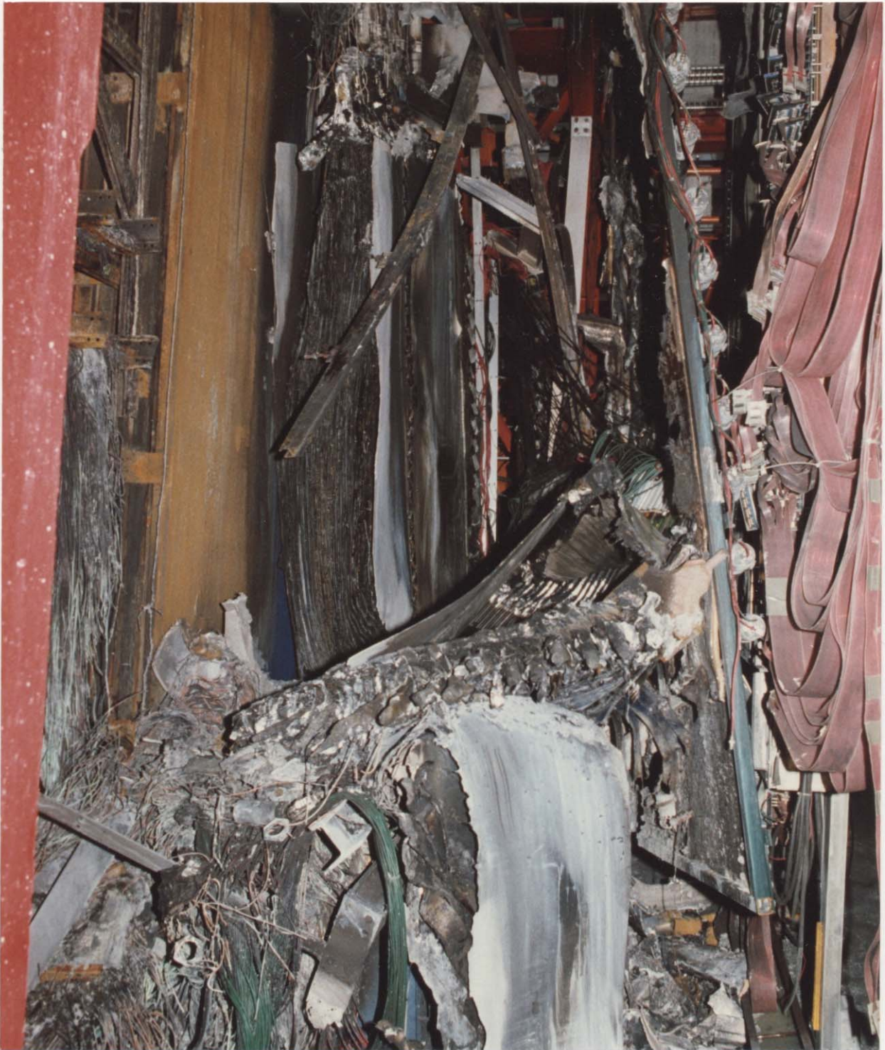
Figure 10. Damage to IEC and HxV. IEC third module and downstream tiebreaker are visible hanging from aluminum framework.
