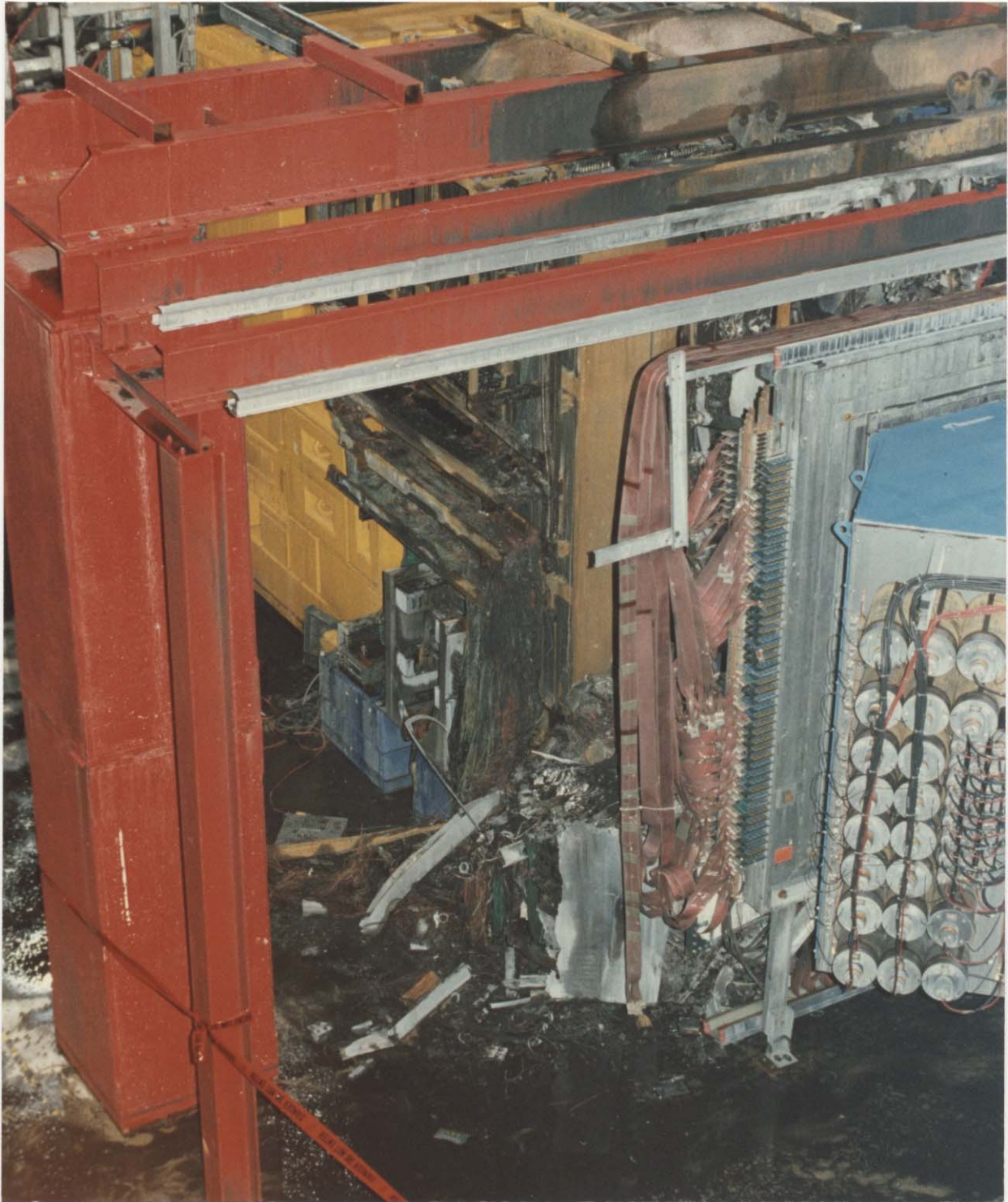
Figure 9. West side of beam line after fire. Note damage to HC, IEC, and support structure, and undamaged ribbon cable on P4.
