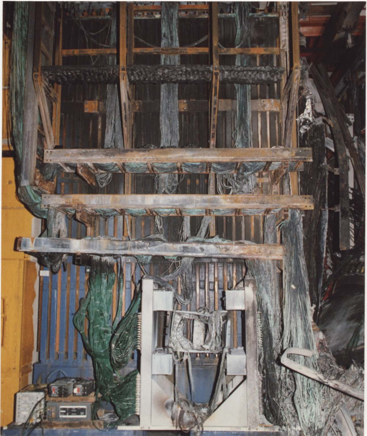
Figure 13. Damage to west side of HC and dynode sum box. Note almost complete destruction of cables on right side of sum box and mostly intact cables on the left.
